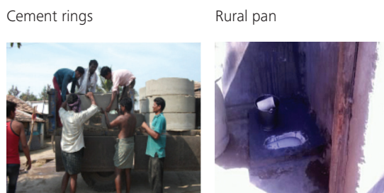
3 feet deep cement ring leach pit with rural pan and brick superstructure
