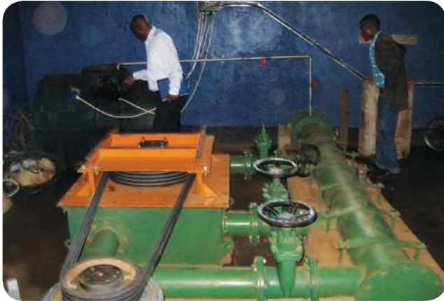
Lower Bondo power house in action
