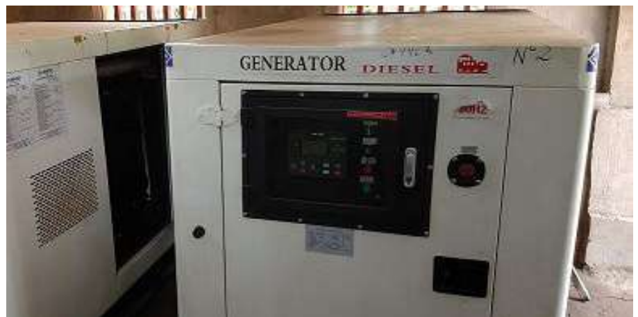
Photo 2 Nyabiheke camp generators
